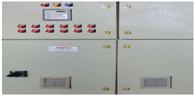
Before- Earlier APFC panel installed. Which is response is very less. Power factor maintain only 0.995. Major gap between active and reactive power.
